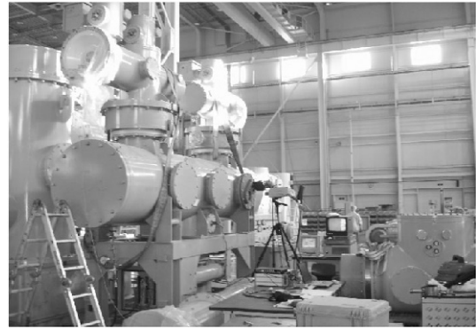
Fig. 3 Gas insulated switchgear
